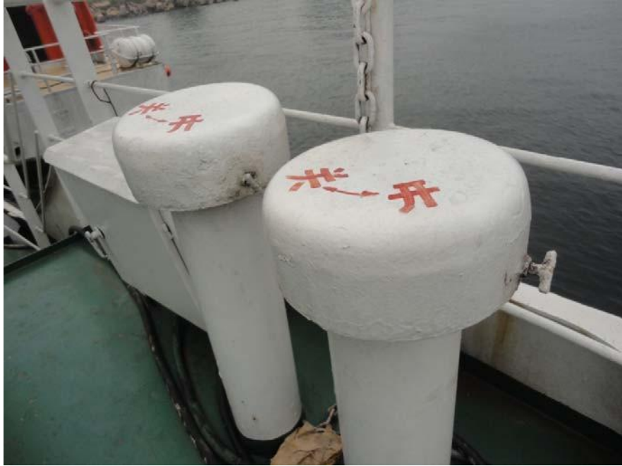
Figure 3.5-15 Type A rotary mushroom-shaped ventilator pipe not allowed for areas described in paragraph 5.2.1
